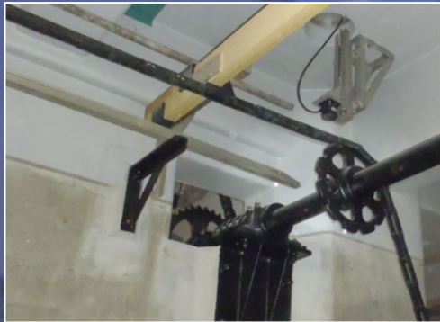
Bearing Section of Sludge Scraper
